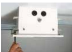
Adjust to ensure ceiling integrity
